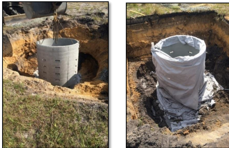
Plates 1 & 2: Soakwell on concrete base lowered into excavated hole and wrapped in geotextile fabric, then backfilled to surface.
